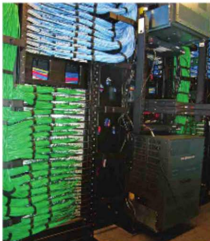
Data center structured cabling plant installation. Photo: PTS Data Center Solutions Inc.
