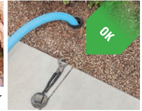
Discharging into a sewer cleanout.
