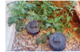
New homes have two sanitary sewer cleanouts. Always pick the one closest to the home.
